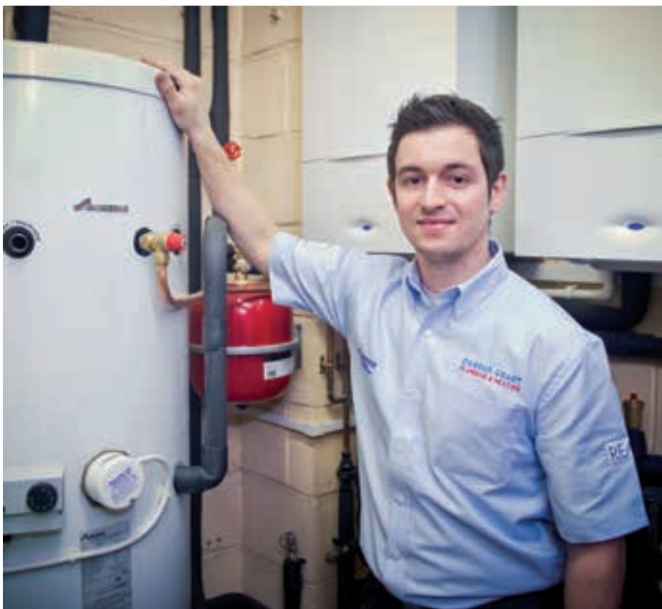
Installer Darren Grant of Darren Grant Plumbing and Heating, installed two Greenstar CDi Classic regular boilers and a Greenstore 210L unvented cylinder to dramatically increase the energy efficiency of a large office in Cardiff.
